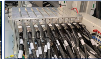
Avionic functional unit
